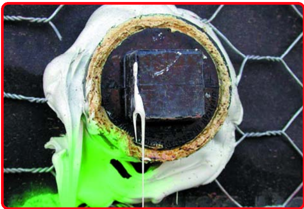
Plumbing Clean Out with Caulking
